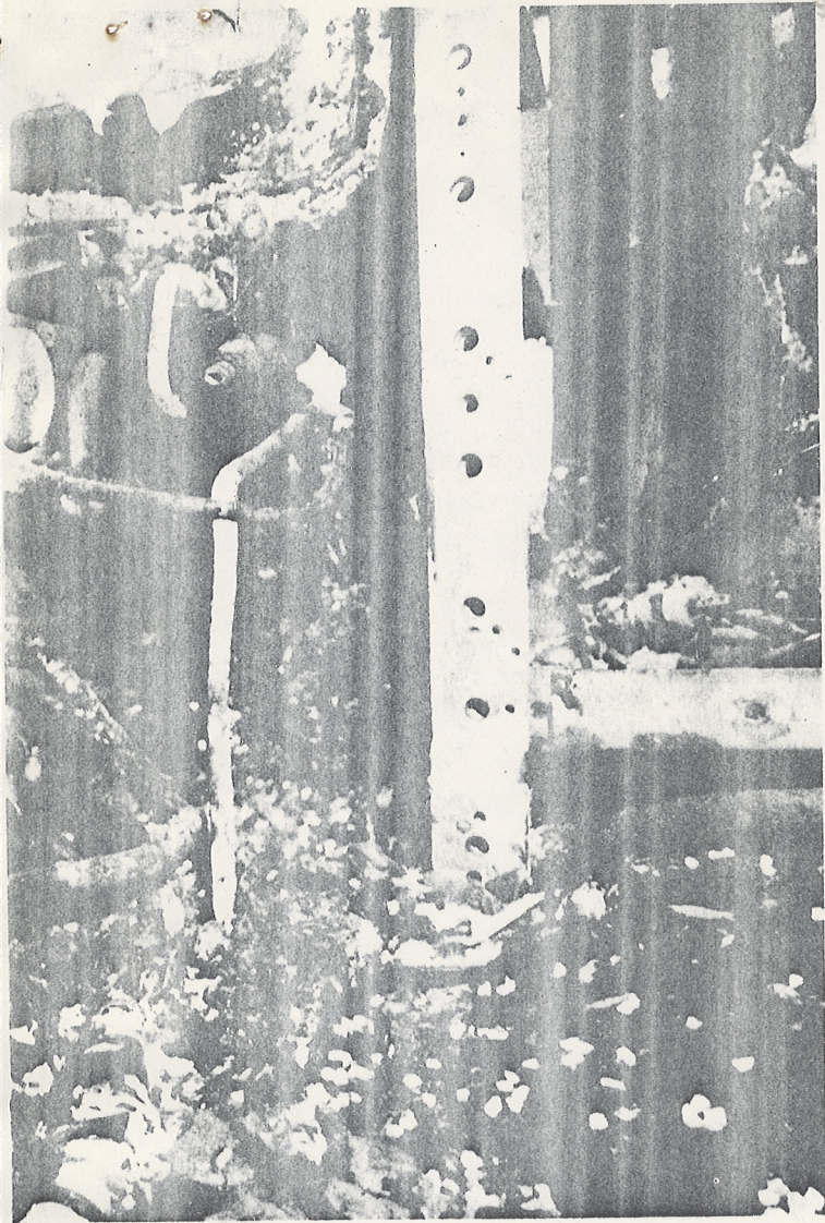
ABOVE: Charred area in spacecraft 012 (essentially the same area shown on page 17) is believed to be the most likely region for the start of the fire. Probable cause is an electrical arc in a power cable. BELOW: View of burned cable.
